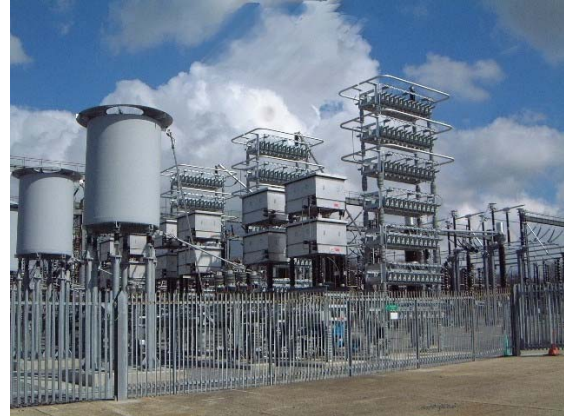
400kV Filter Resistors
