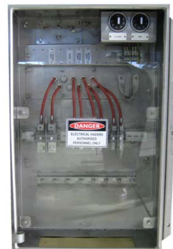
IP56 cable termination compartment showing thermostats, high temperature cable, earthed brass gland plate, cable sheath termination bar, perspex shield, and resistor labels
